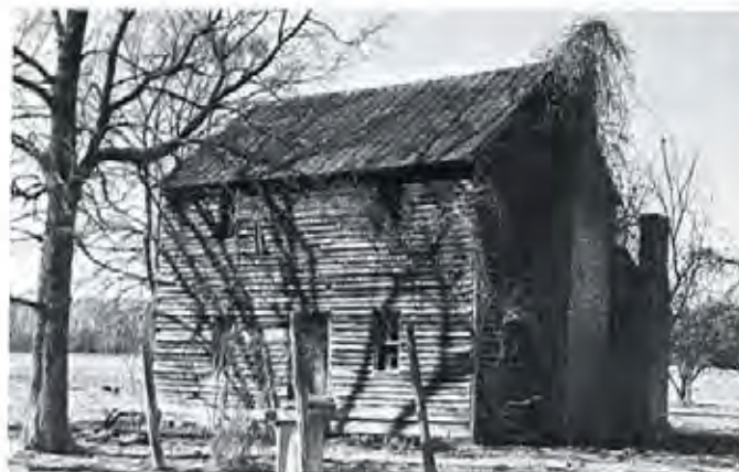
Figure 19. Matthias Phifer Log House, vicinity of Third Creek Church, Rowan County, North Carolina, built about 1800. This small Continental plan dwelling displays a transitional two-bay second floor, three-bay ground floor combination. The shed element with independent chimney is original and common in the locale.
