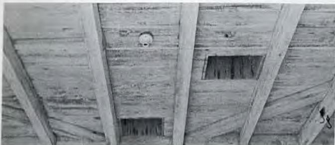
Figure 14. Ventilation chutes in front porch ceiling, "Sloop Point," Pender County, late eighteenth century.
