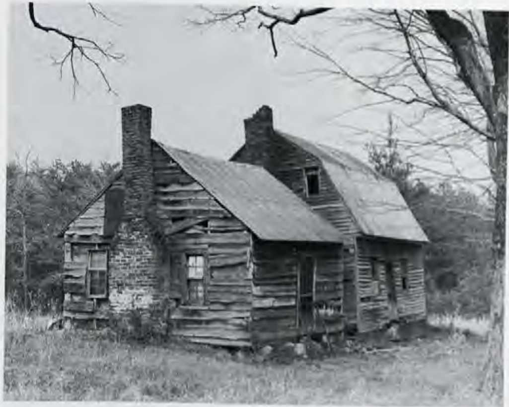
Figure 1. Manlove Wheeler House, late eighteenth century. Though houses of this type were once common in eastern North Carolina, only this rare example survived until recent times in Guilford County. This 1972 photograph shows the dilapidated structure with a later addition and replacement chimneys. The house was eventually demolished, further obscuring the record of the county's eighteenth century architecture.
