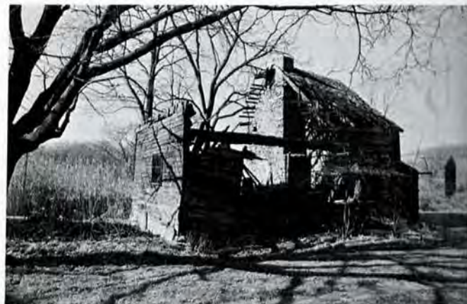
Figure 4. Pott Log House, vicinity of Lobachsville, Berks County, Pennsylvania, built mid-eighteenth century. In ruins, the Pott House provides a rare cross section of the formal features of a Continental plan house including a two, rather than three, room plan and large central fireplace.
