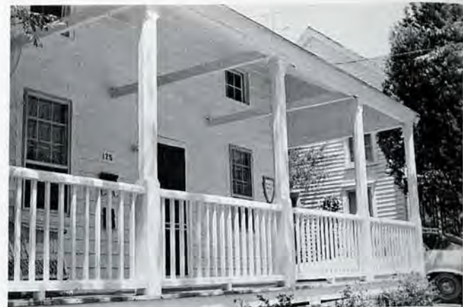
Figure 13. Attic ventilation window above the ceiling joists of the Jesse Piver House porch in Beaufort.
