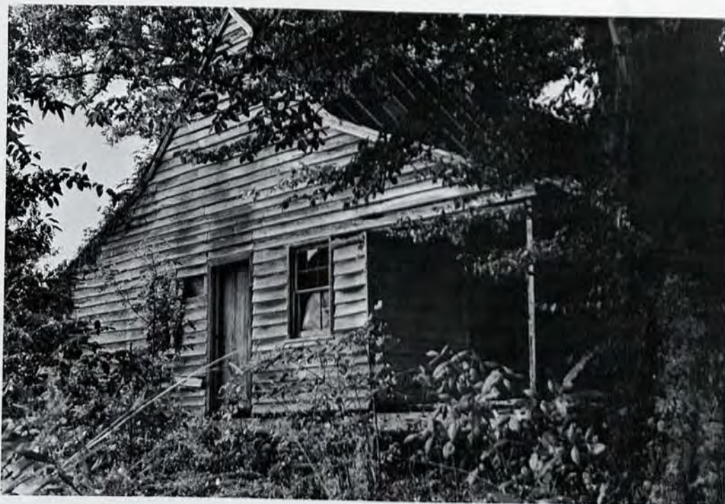
Duplin County house in ruin.
