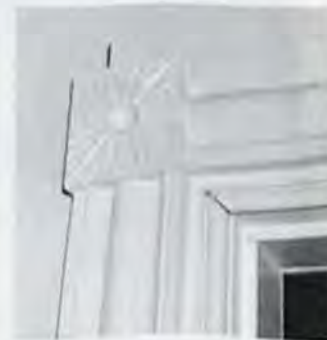
Figure 10. Low House, located in the heart of Guilford's German settlement. Interior detail shows Greek Revival style door surround with unusually treated corner block. Other details are fully developed Federal style.
